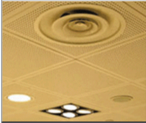
Mounted into ceiling tile
