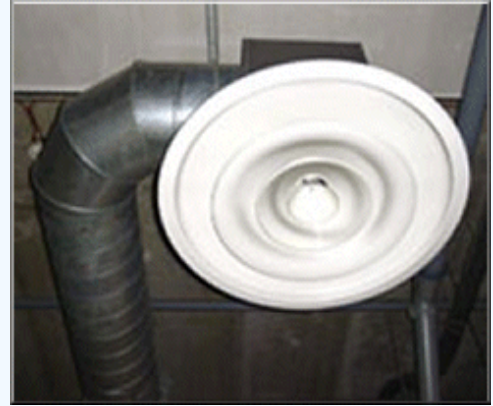
Mounted directly onto duct
